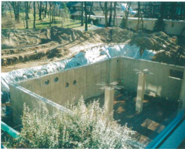
The underground central chiller plant, shown during construction, was integrated with a primary-secondary pumping system.
